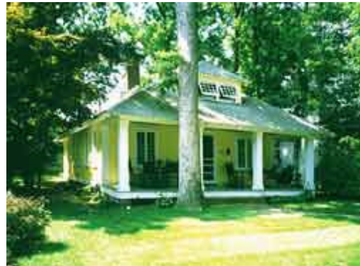
Unacceptable: Insufficient foundation height. Otherwise acceptable.
