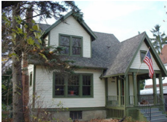
Unacceptable: Porch too small, iron handrails are not acceptable, stem wall foundation exterior not finished
